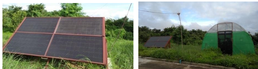
Figure 3.7. Solar Power System
